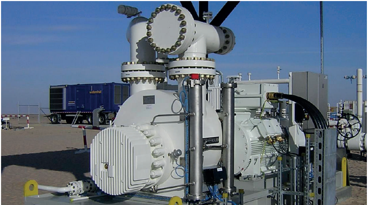
Multiphase „Boosting in Libya“
