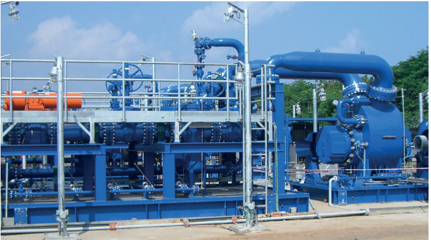
Onshore Terminal in India
